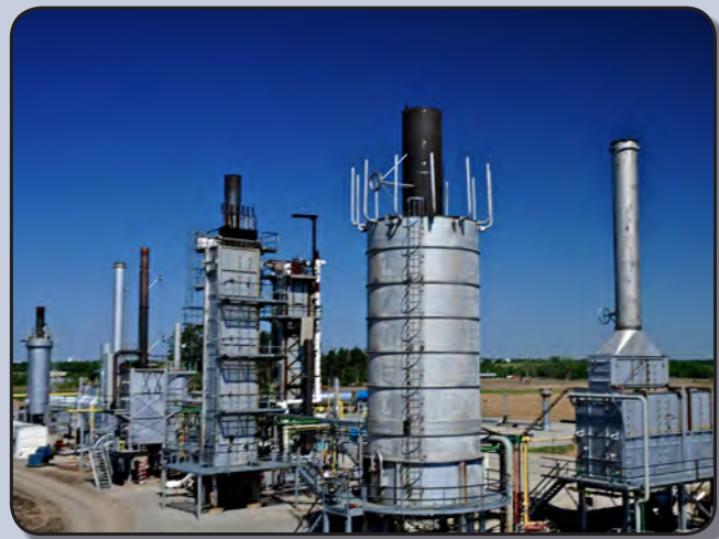
ZEECO Combustion Research and Test Facility
