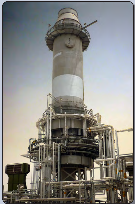
ZEECO Nitrogen Bearing Waste Thermal Oxidizer
